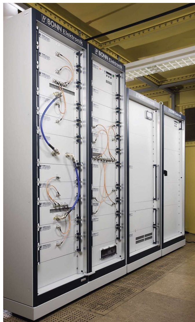
FIG 2 The amplifiers are accommodated in a central, shielded room and can be assigned to the test chambers as required.
