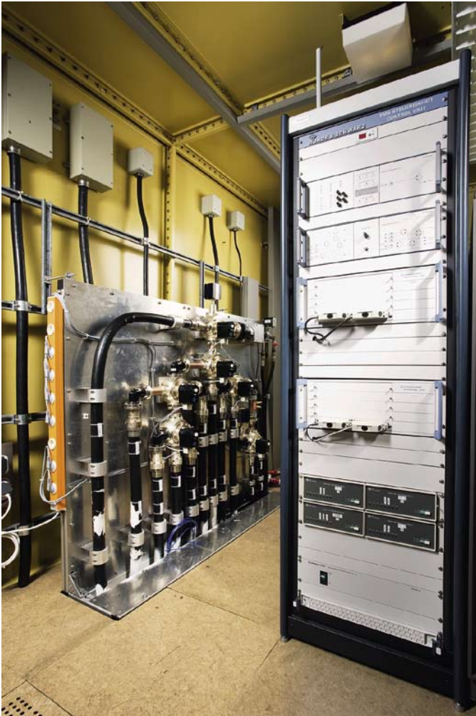
FIG 4 Rack for controlling the amplifier switching in the amplifier room, and in the background the associated RF power switch unit.
